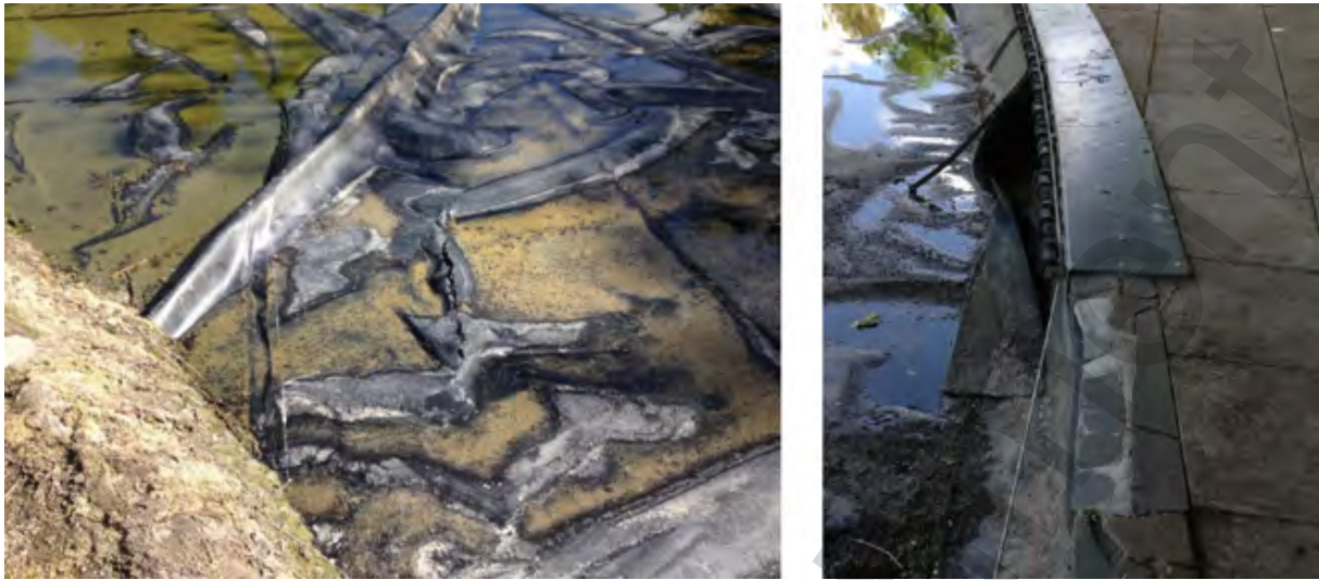
Figure 4.1: Deterioration of existing liner on pond bed and liner separation from pond wall
